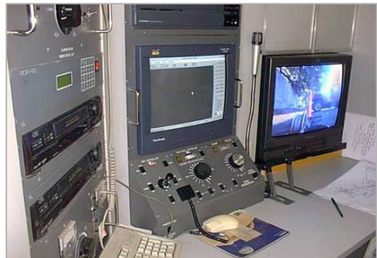
Inside of TV Inspection Truck
