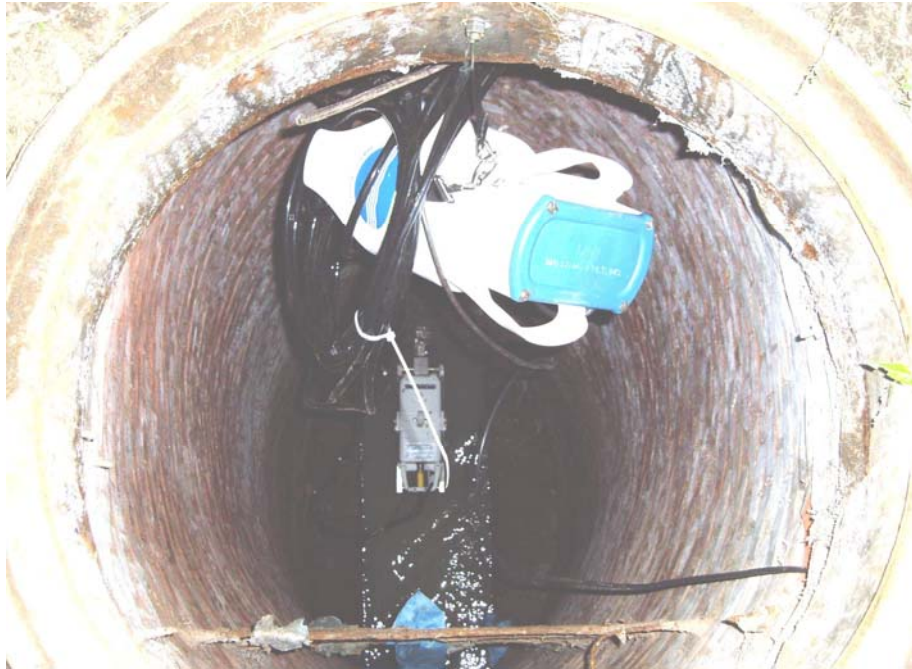
The above photo shows a typical wastewater meter installed in a sewer manhole. The data recorder is suspended at top of manhole and the depth/velocity sensor is mounted near the wastewater flow at the bottom of the manhole.
