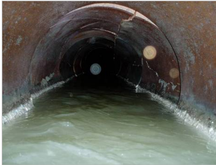
Example of sewer needing rehabilitation
