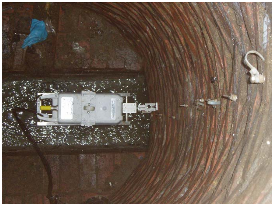
The above photo is a close-up of the depth/velocity sensor mounted near the wastewater flow.
