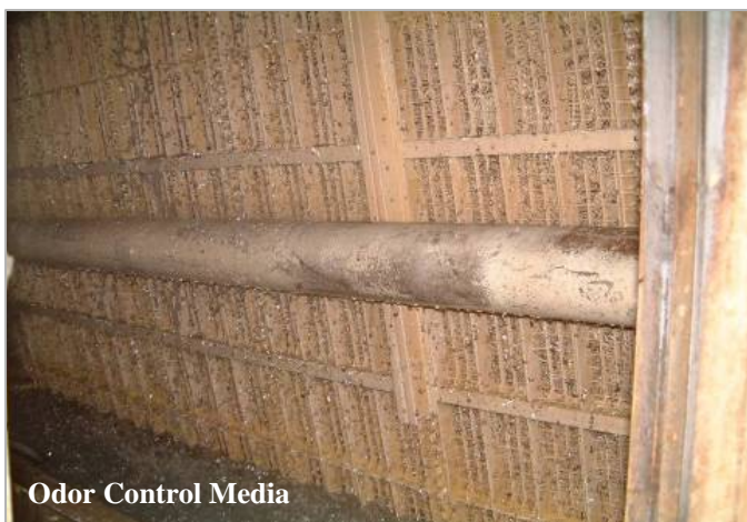
The photo at left shows the odor control media typical of all three older remote headworks – Chelsea Creek, Columbus Park and Ward Street. The odor control systems are in need of replacement.
