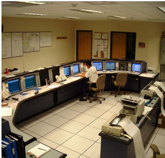
MWRA Operation Control Center
