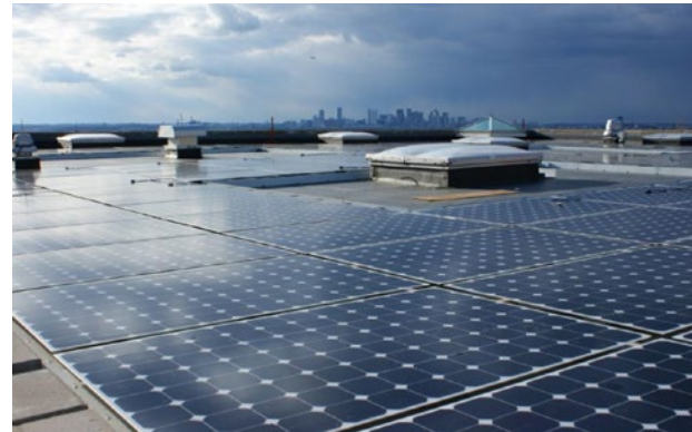
Solar Panels at Deer Island – contribute to renewable energy generated and used on-site.
