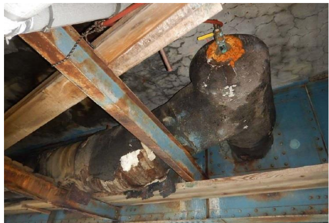
Figure 9 - Insulated Pipe at Bend and Twisted/Deteriorated Support Beams at Span 5
