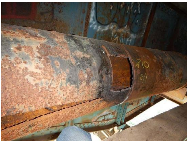
Figure 8 - Pipe Blowout Area Span 10 with Coupon Cutout
