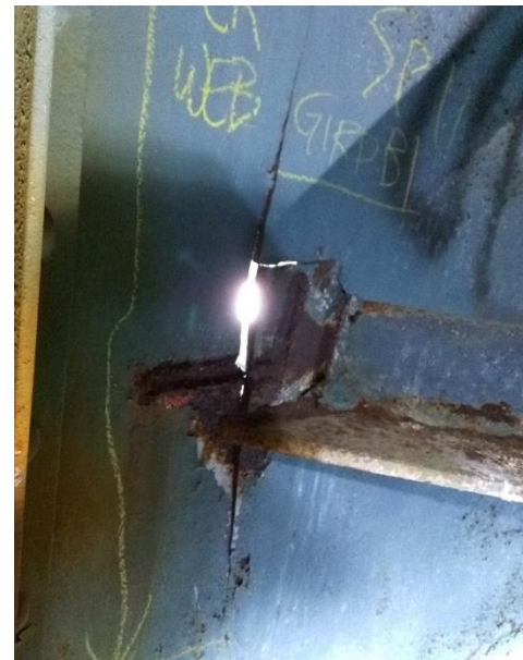
Figure 14 - Cracked Girder Web Span 11
