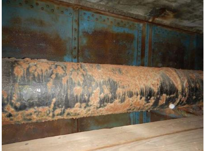
Figure 7 - Typical Exposed Pipe Condition
