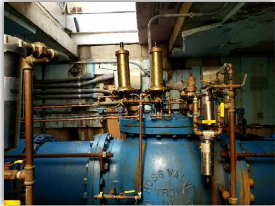
W14 Nonantum Road PRV Vault
