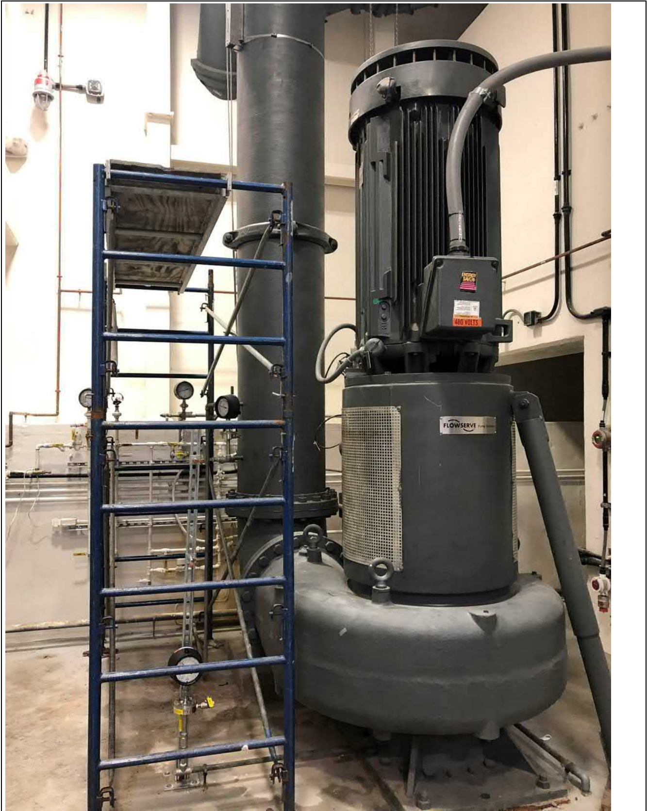
Figure B.1: Dry weather pump, pump 4, suction and discharge pressure gauges shown
