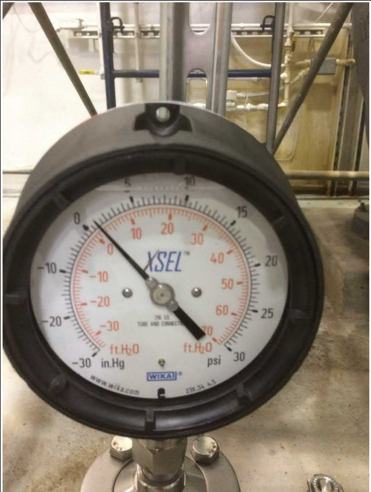
Figure B.5: Dry weather pump, pump 4 suction pressure gauge
