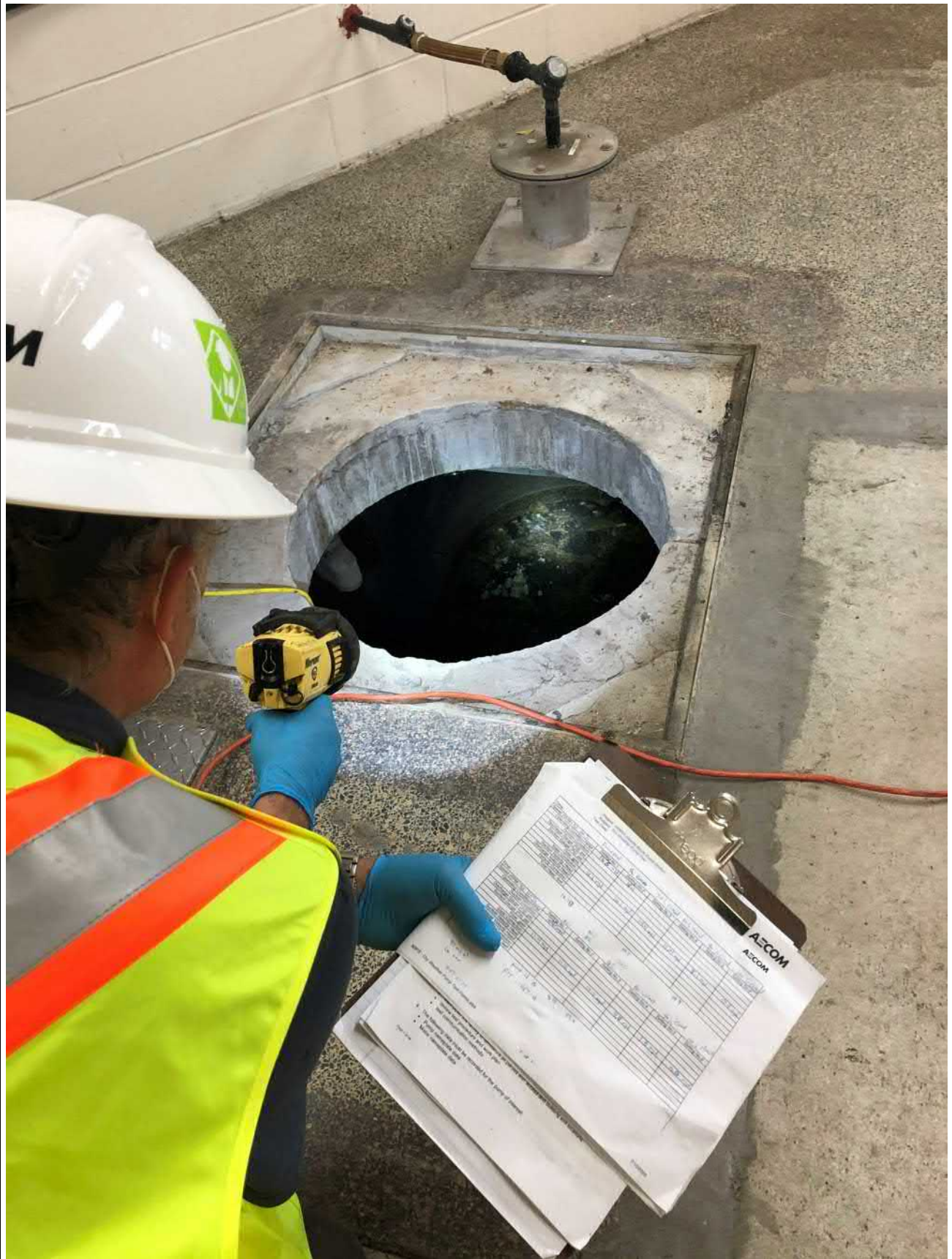
Figure B.7: Wet well drawdown test, access port used for observation
