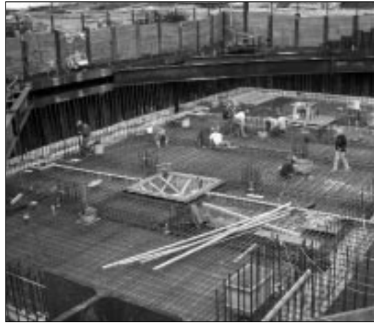
The left photo shows a structure that resembles construction of a similar, above-ground facility; on the right, typical below grade concrete work.
