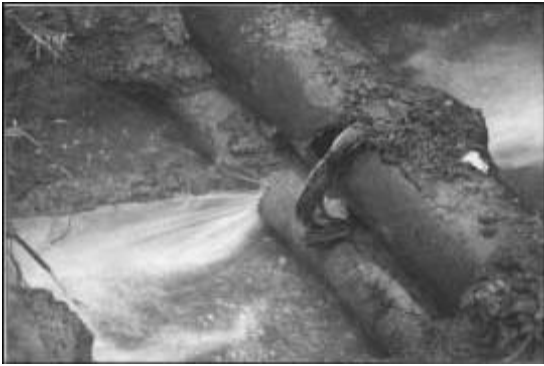
Figure 6. Leaking water pipe next to sewer pipe
